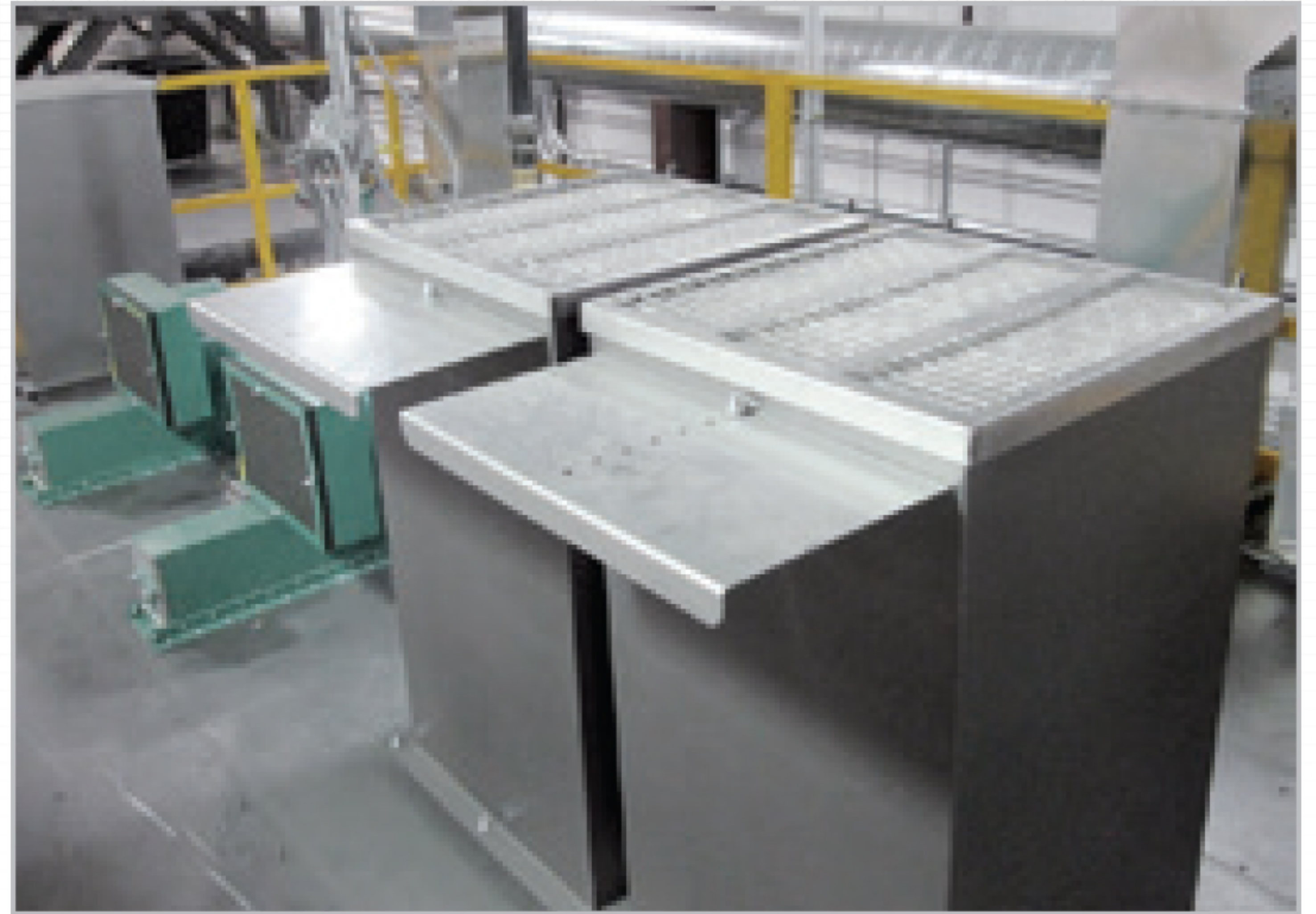
Filtered make up air and burner air to reduce cross-contamination or re-contamination
